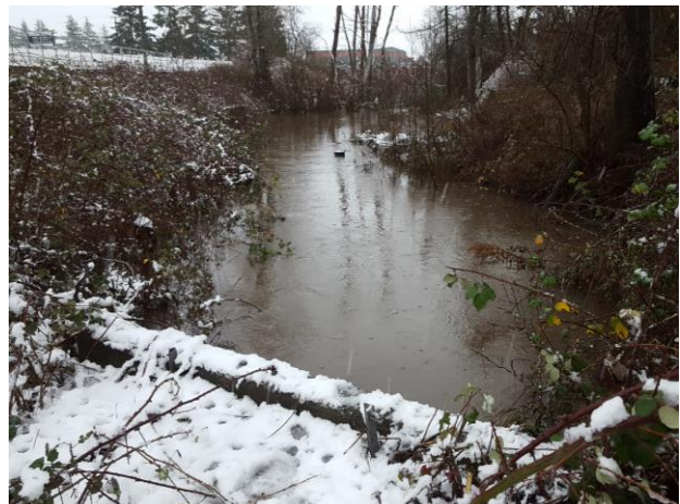
Photo 2: Culvert Inlet @ 2:14 pm Recorded Water Level – Surcharged and staff gauged observed just below surface
