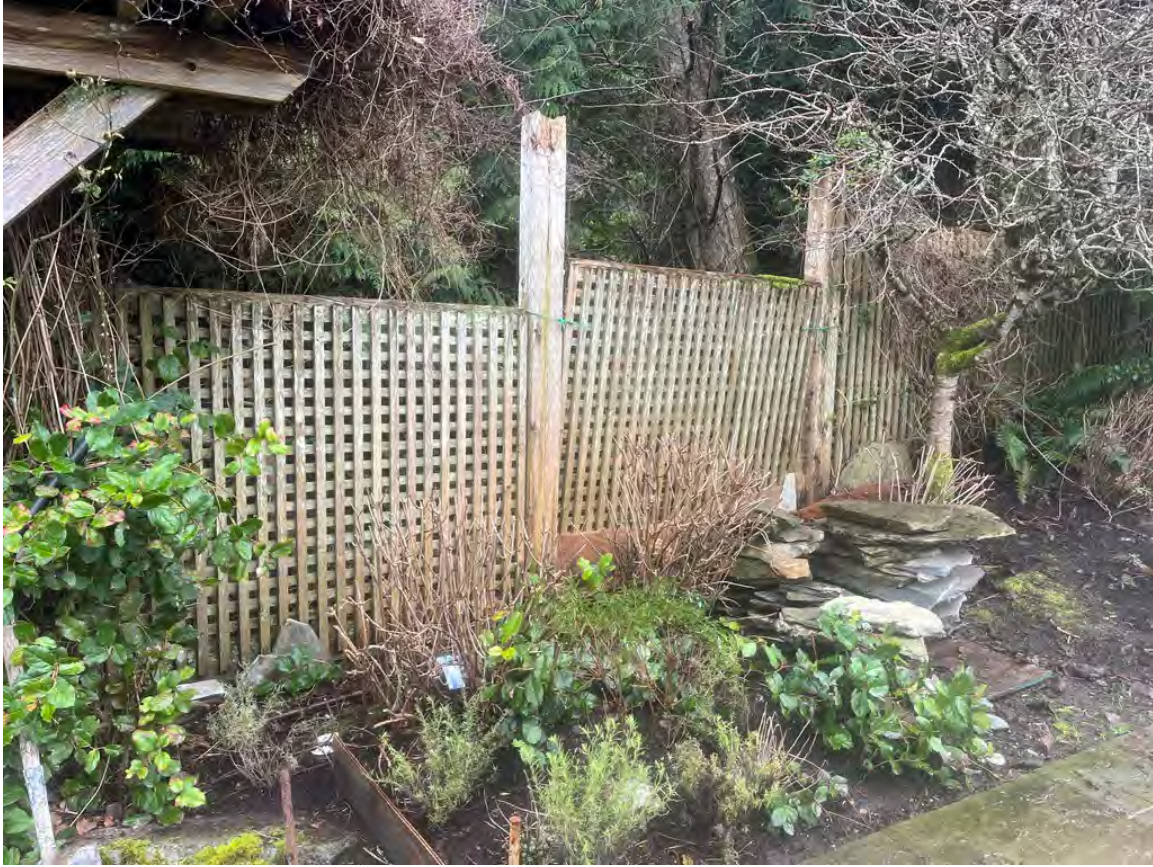
Figure 16. The eastern fence will be replaced as it has reached the end of its structural lifespan.
