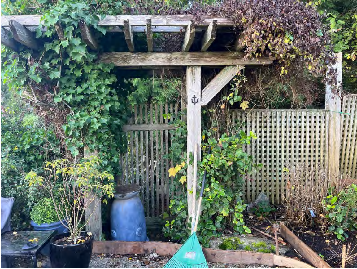
Figure 15. Looking east to the gate in the eastern property fence. The gate provides access to the municipal trail, the latter a public access to the shoreline. The gate and fence will be replaced as they have reached the end of their structural lifespan.
