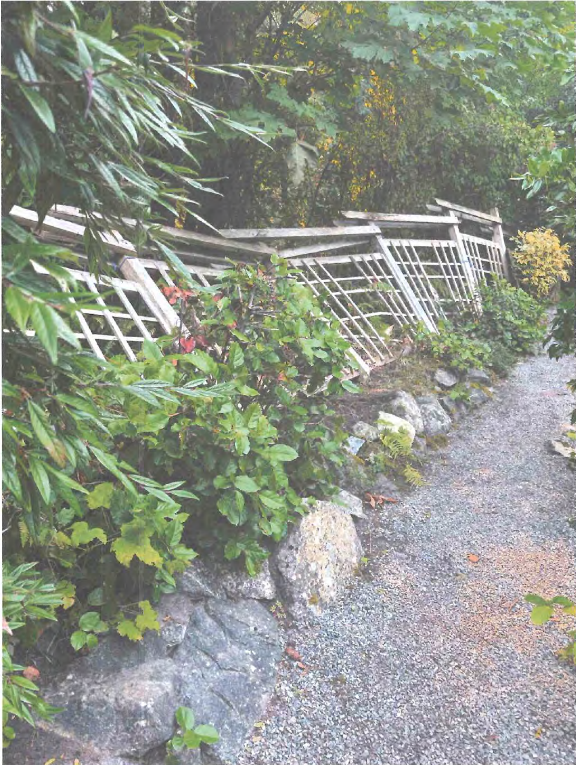
Figure 17. The eastern fence will be replaced as it has reached the end of its structural lifespan.
