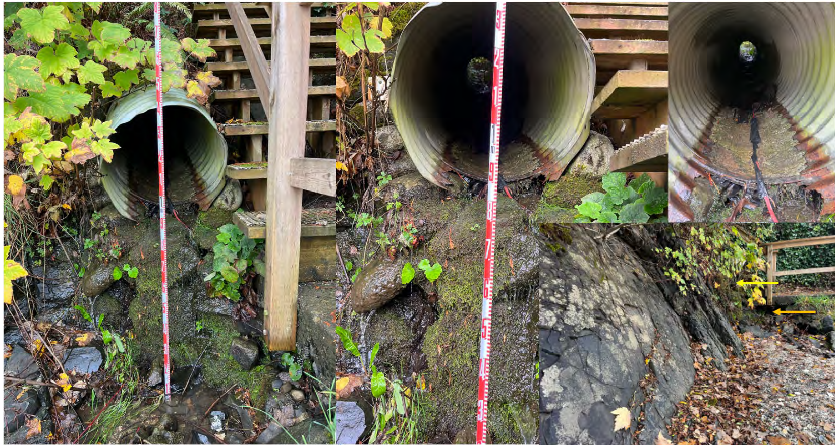
Figure 2. Discharge end of CSP culvert in the municipal shoreline access trail. The CSP culvert has disintegrated in the lower segment, with stormwater discharge flowing under the culvert (inset images on right hand side of figure). The invert of the culvert's discharge is 0.9 m above the upper intertidal shoreline. The High Water Mark of the shoreline (orange arrow) lies below the culvert's invert (yellow arrow). The culvert has a slope of ~35%. This culvert discharges directly onto the marine shoreline's upper intertidal. Thus, it is the opinion of the authors that this drainage ditch is not subject to the RAPR or the Water Sustainability Act . Note the municipal public access, wooden stairs leading to the shoreline (far right hand side of photograph).
